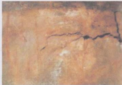
Gambar 2.9 Stress Corrosion Cracking
