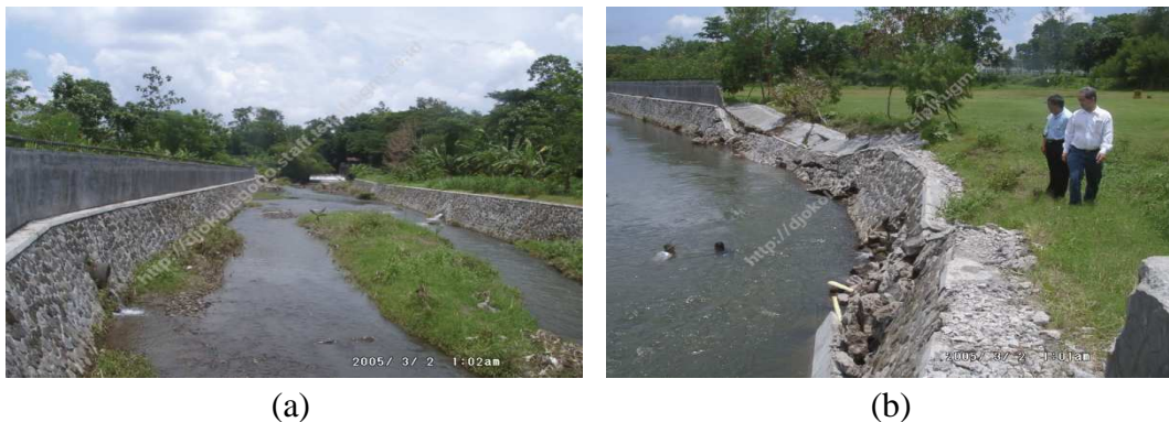
(a) (b) Gambar 2.2 Kegagalan konstruski dinding penahan tebing sungai (Photo courtesy: Djoko Legono)
