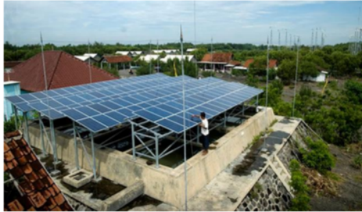
Figure 3. Solar panels in Pantai Baru hybrid power plants
