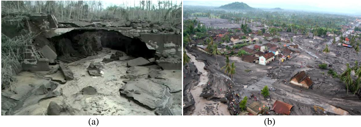
Figure 1. (a) A Damage Check dam in Putih River, (b) Deposited Sediment in Salam Sub District, Magelang Regency
