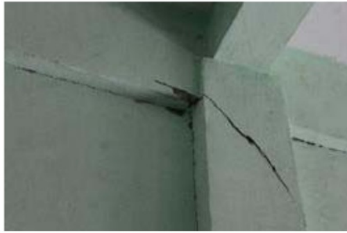
Figure 13. Damage to column components
