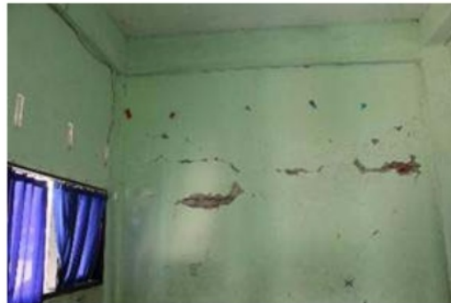
Figure 14. Horizontal cracks occur on the wall
