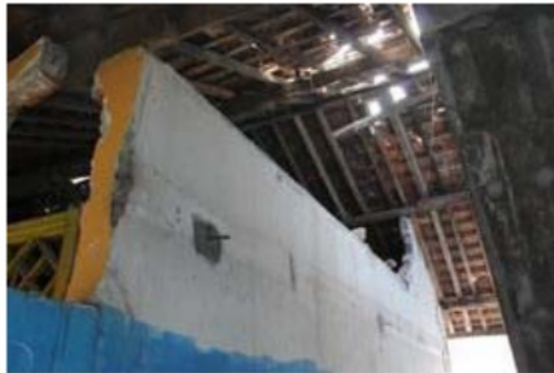
Figure 12. Damage to the roof frame structure
