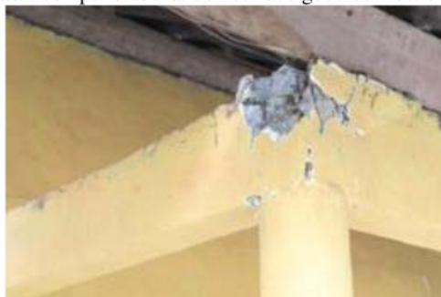
Figure 11. Damage to beam joints and columns
