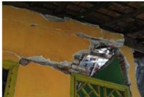
Figure 10. Damage to wall components that do not have good connections with doors and windows
