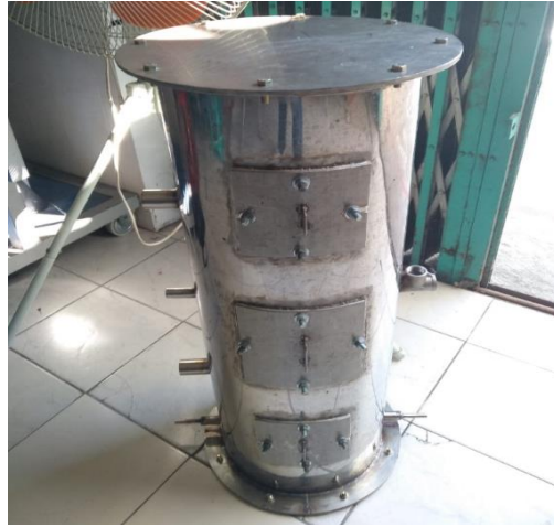
Gambar 3. 6. Tangki solar water heater belum terpasang glasswool dan aluminium.
