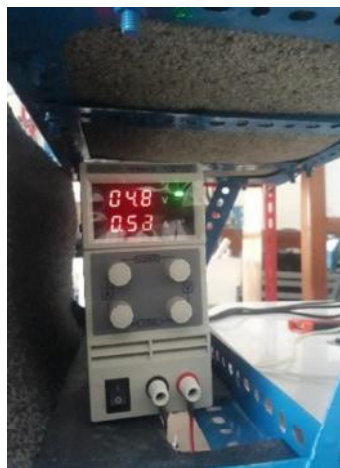
Gambar 3. 17 DC power supply
