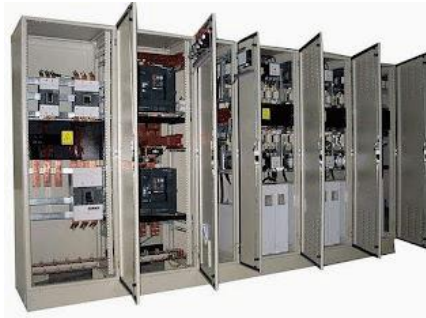
Gambar 4. Medium Voltage Main Distribution Panel
