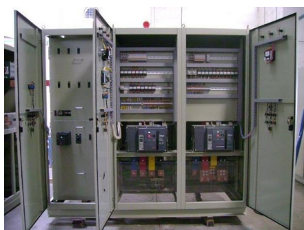
Gambar 6. Low Voltage Main Distribution Panel
