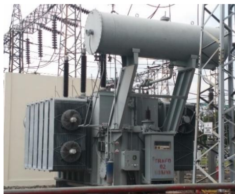
Gambar 2.1 Transformator Daya 150 kV
