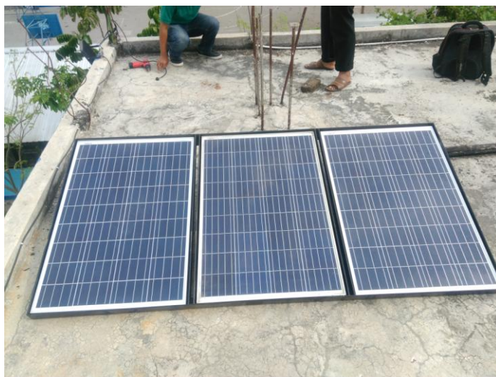
Gambar 4.4 : Panel surya Solar Home System MBS
