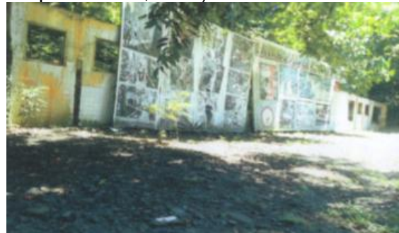
Figure 4. Present Day Abandoned Clinic where the emergency hospital was raided by New People’s Army happened on April 1985. (Photo taken by researcher last September 13, 2014)
