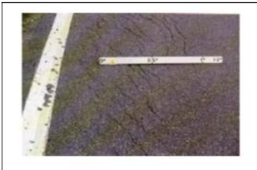
Gambar 2.35 Patah Slip ( Slippage Cracking )
