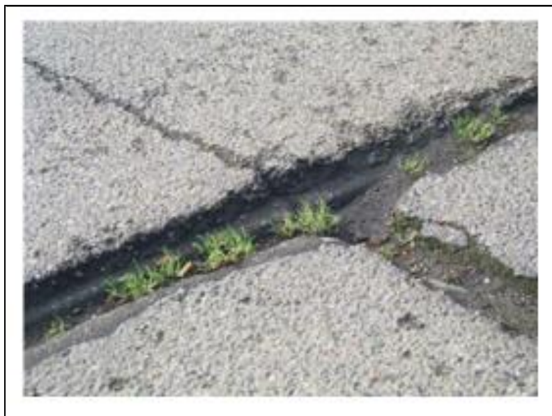
Gambar 2.17 Retak sambung ( Joint Reflect Cracking )
