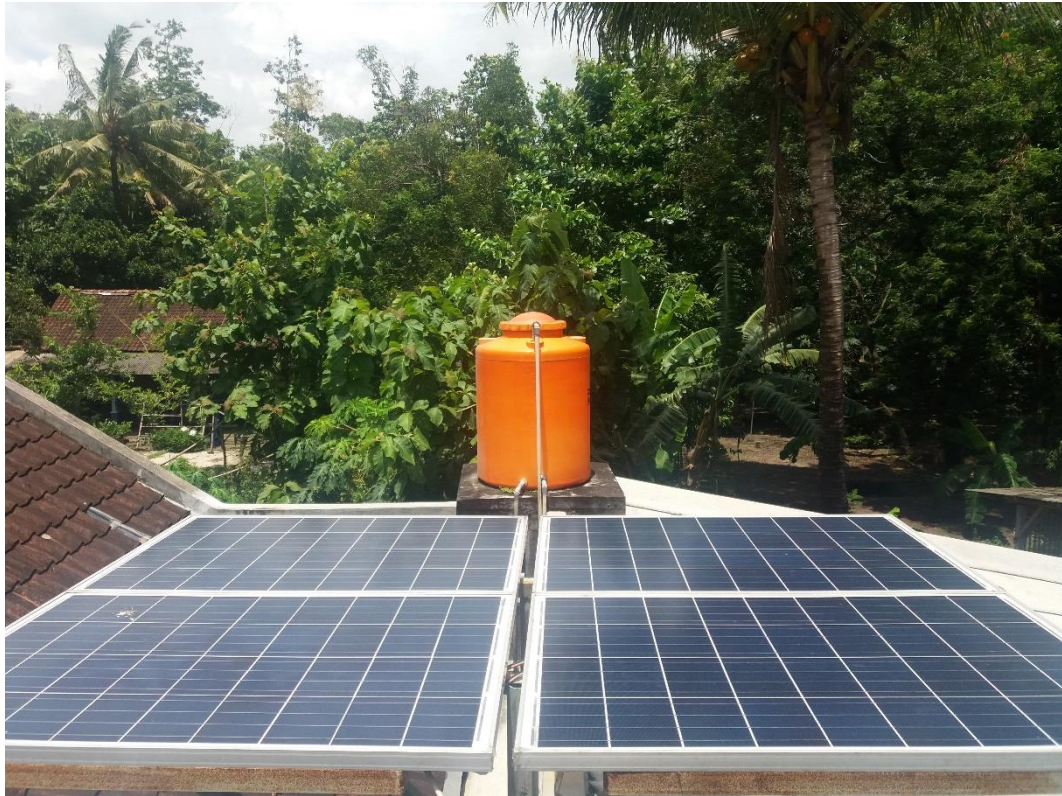
Panel Surya Terpasang
