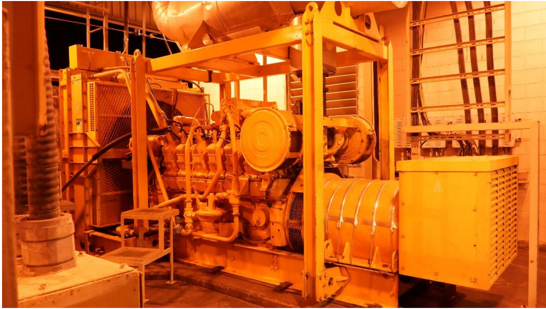
Lampiran 2. 3512 Caterpillar Gas Engine Generator
