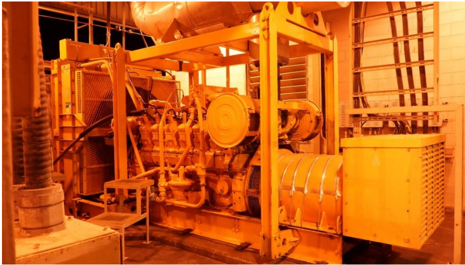
Gambar 2.12. 3512 Gas Engine Generator
