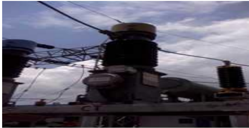
Gambar 2.4 Current Transformator (CT)
