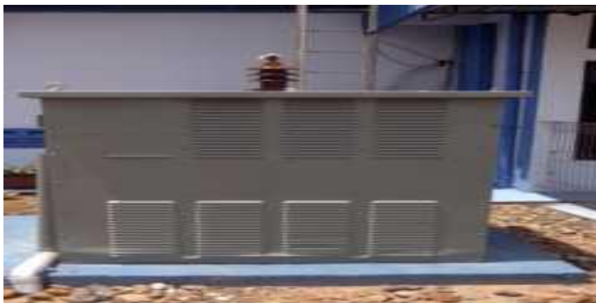
Gambar 2.3 Neutral Grounding Resistance (NGR)
