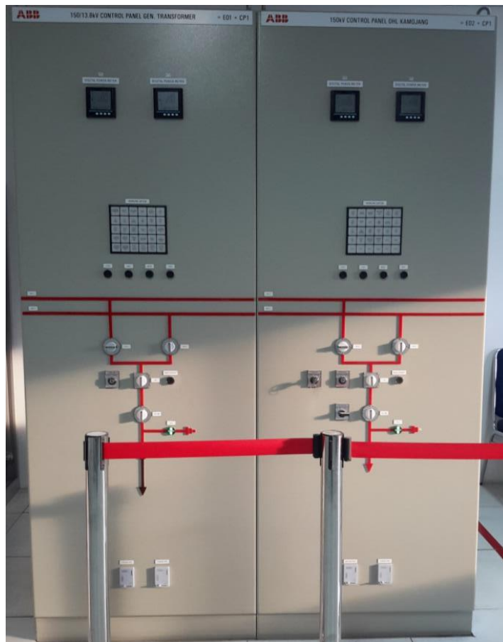
Lampiran 11. Panel Kontrol Transformator Daya KMJ Unit 5
