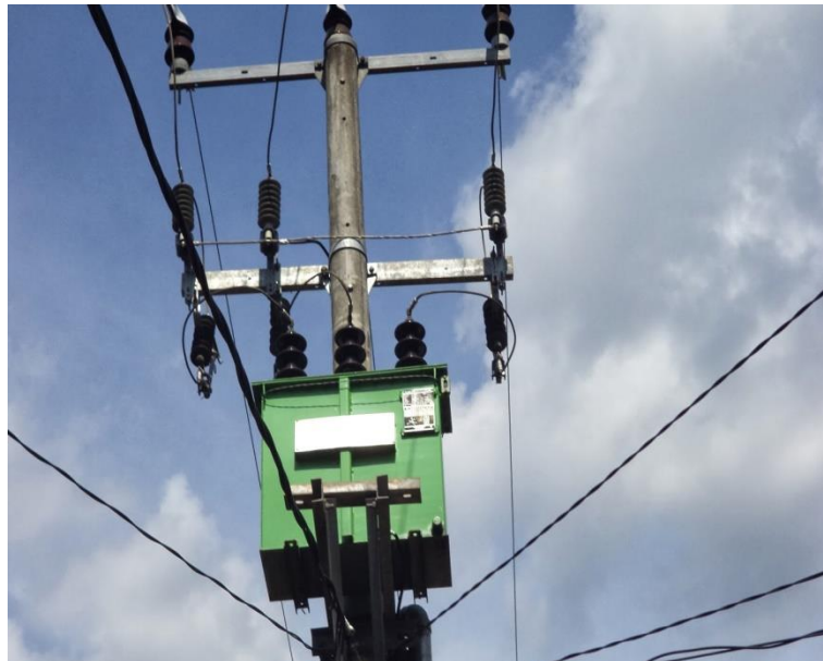
Gambar 2.14 Trafo distribusi 3 fasa
