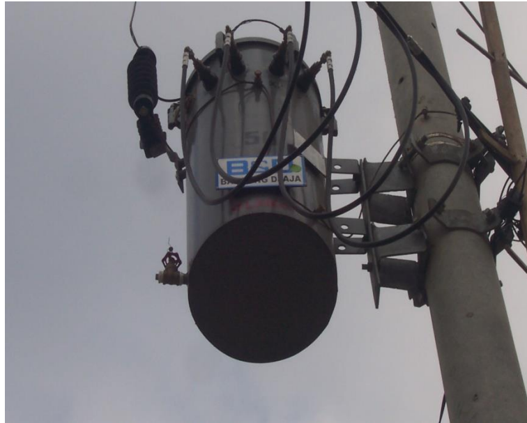
Gambar 2.14 Trafo distribusi 1 fasa
