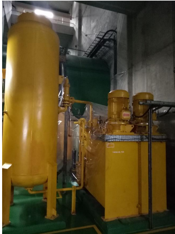
Gambar 2.12. Air/Oil Receiver dan Sump Tank (Sumber : PLTA PB SOEDIRMAN, 2017)
