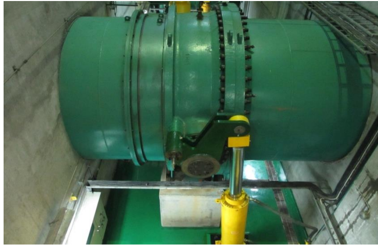
Gambar 2.3. Main Inlet Valve (Sumber : PLTA PB SOEDIRMAN)
