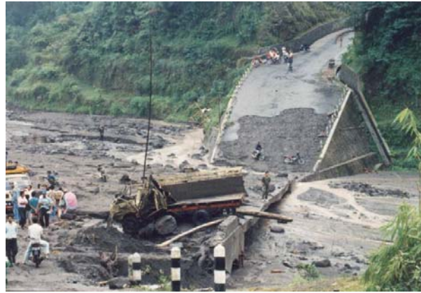
Photo 1.3 Damages at Kemiri Bridge on Boyong River in 1994 caused by a debris flow (Photo courtesy Adhy Kurniawan)
