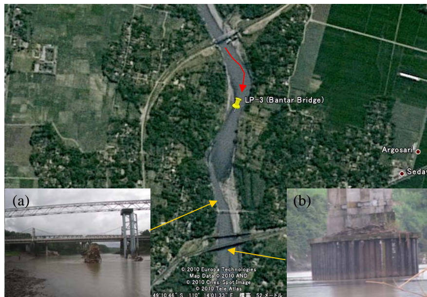
Photo 2.3 (a) The Bridges in Bantar and (b) a foundation is exposed by the riverbed degradation. The photos were taken in December 2008 (Source: Google Earth, 2010)
