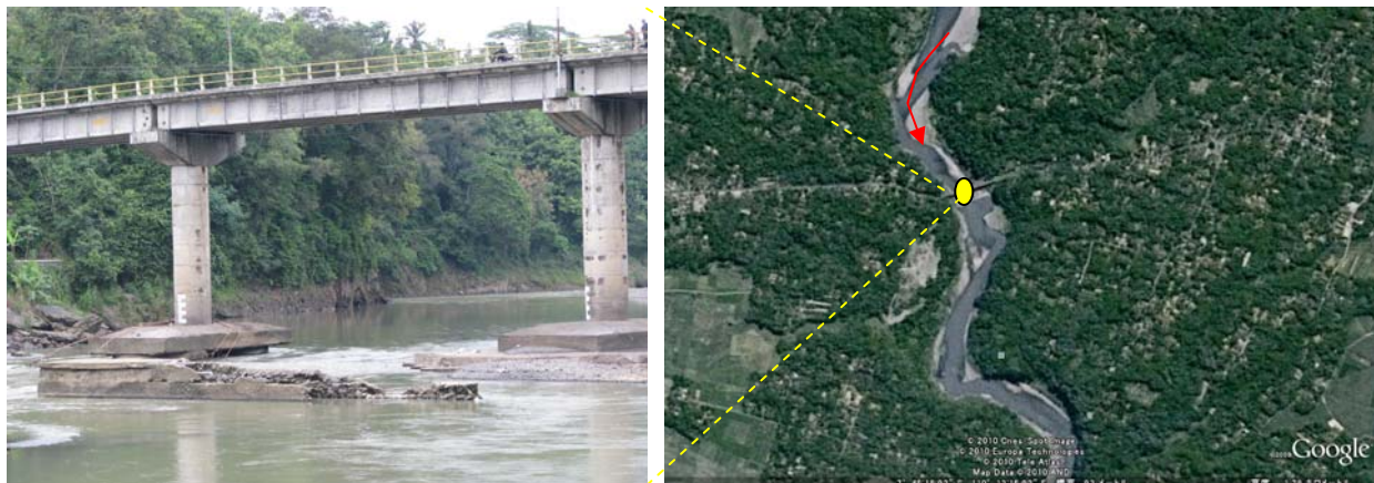
Photo 2.4 The Kebon Agung Bridge. The foundation is exposed by the riverbed degradation. The photo was taken in December 2008 (Source: Google Earth, 2010)
