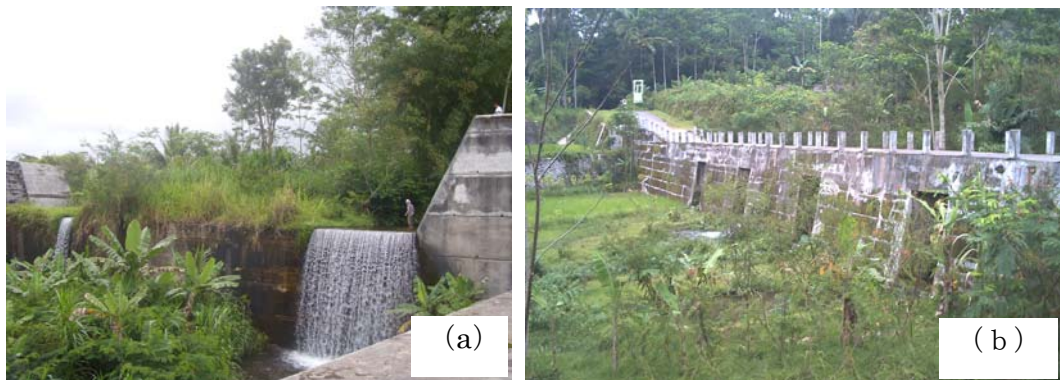
Photo 3.3 Existing of sabo works on slopes of Mount Merapi. (a) A Check dam functioned as an intake and a sand pocket on Blongkeng River (BLD1). (b) A Consolidation dam on Putih River functioned as a bridge (PU-C8A) (Photos were taken in December 2008)
