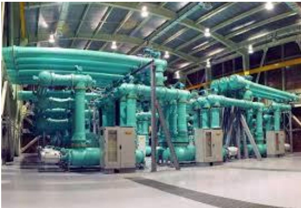
Gambar 2. 9 Gas Insulated Substation
